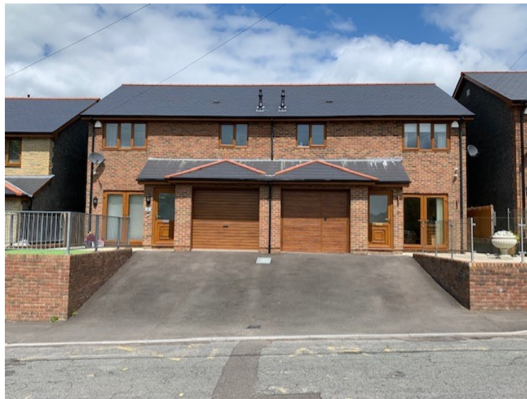
Photograph 15 : showing driveways fronting 2-3 Rhys yr Ysgol – width reduced from that indicated on the approved plans. Individual driveways capable of accommodating one vehicle rather than the two indicated on the approved layout plans..
